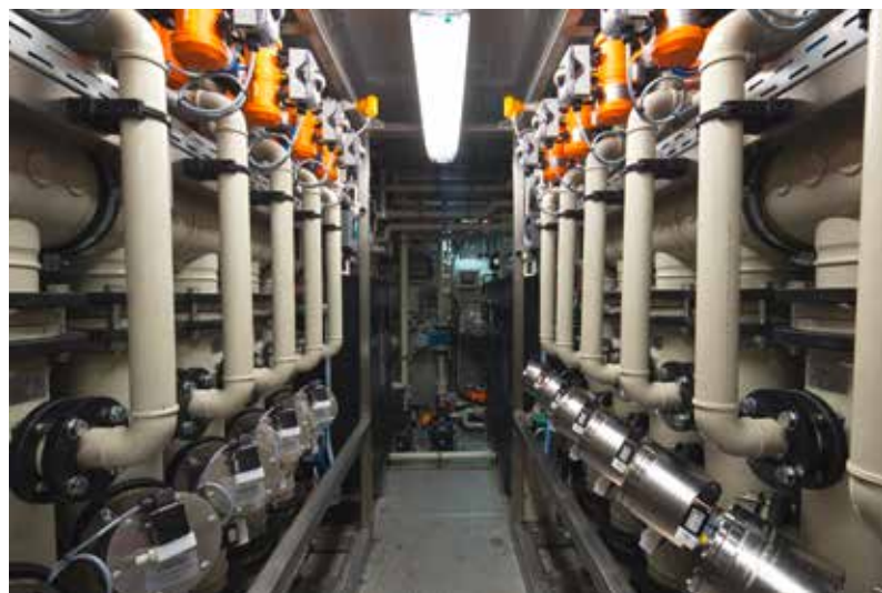
Redundantly equipped ultrafiltration in the OilPaq container
